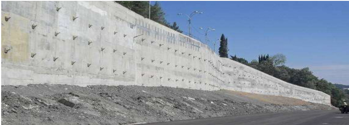
Pile anchor landslide protection structure at the interchange in the area of the city of Sochi (© Rosasfalt)
